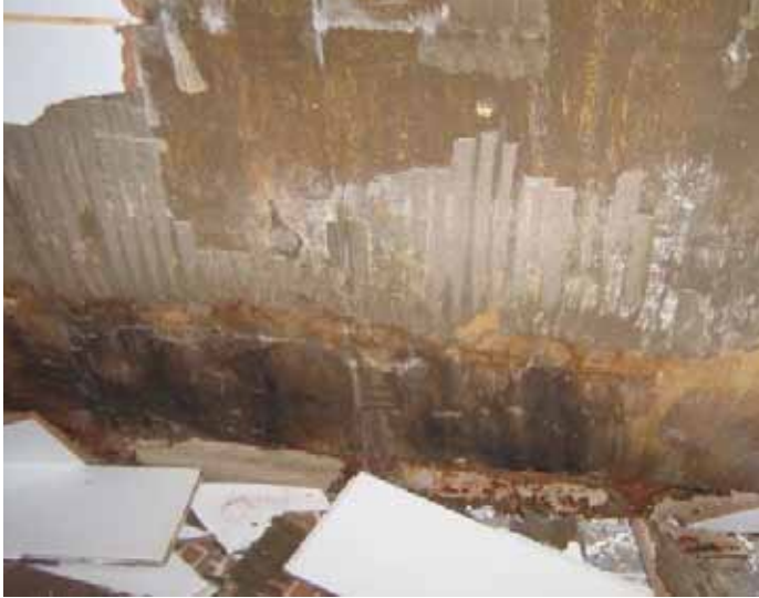
▲ This happens when water seeps behind ceramic tiles
